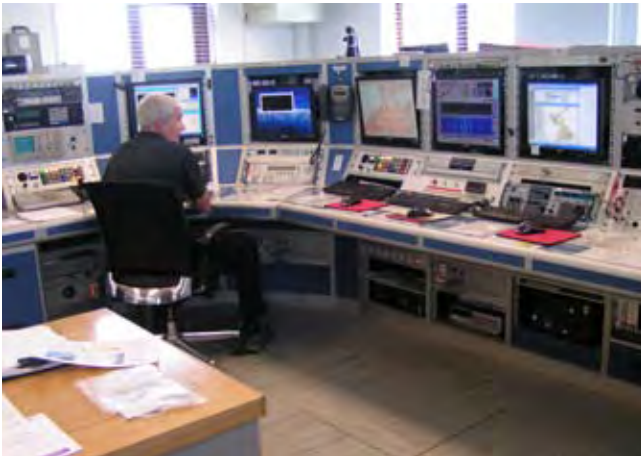
Figure 4: Baldock Radio Operations Centre with Roke SRDF (image courtesy of Baldock Radio Station)
